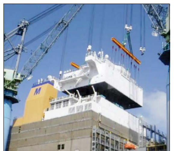
At the NASSCO shipyard in San Diego, the house top of the Ro/Con Lurline including the navigational bridge, is lowered into place beginning the final phase of construction. The ship was 85% complete on May 3.
